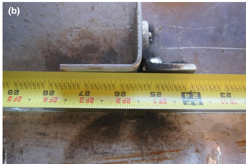
Figure A12. Detail of the position of the upper (a) and lower (b) fin supports with measuring tape. Both measurements are shown from the top of the mast (in inches).
